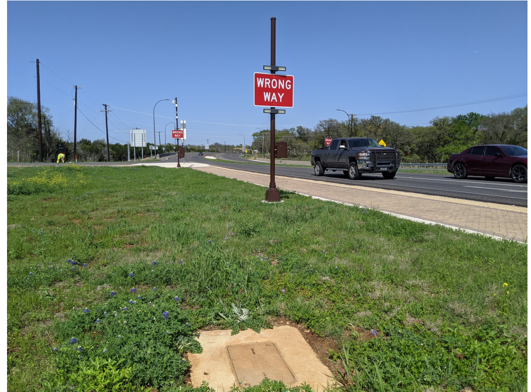
Wrong Way Vehicle Detection System (WWVDS)
