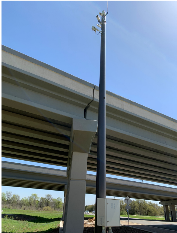
Closed Circuit Television (CCTV)
